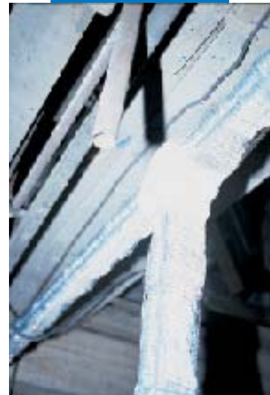
Deteriorated concrete structure
